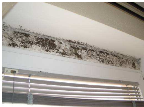
Figure 6: Mould on a thermal bridge (M. Tomšič)
