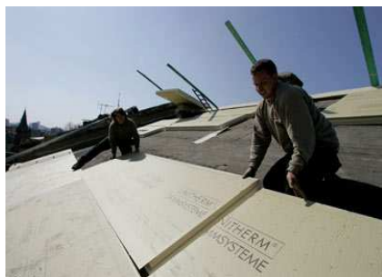
Figure 11: Workers installing thermal insulation on the roof of a building in Frankfurt, Germany ( home.howstuffworks.com )
