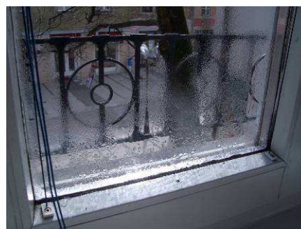
Figure 17: Condensate on internal surface of glazing as a consequence of a too high level of relative humidity in the room (M. Tomšič)
