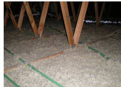
Figure 10: Rockwool Blow in - ceiling insulation ( www.igloo-insulation.co.nz/107842/html/page.html )
